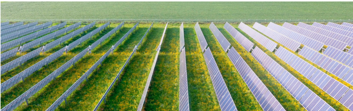
Figure 20. One of Dairyland Power Cooperative's community-hosted solar sites colocated with pollinator gardens.
